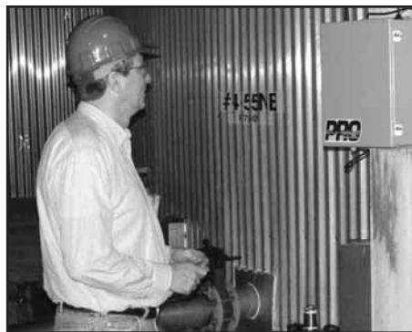
Installation of the Communication Module in the CASCO Tank Farm.
