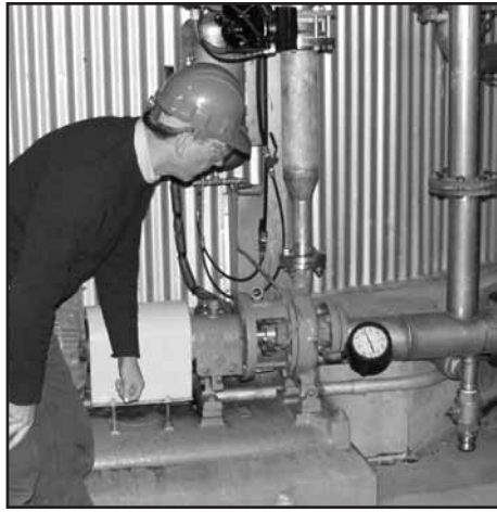
Pumps not monitored by PROsmart still require periodic visual inspections.
