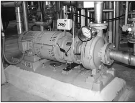
PROsmart Data Monitor installed on a 3196 MTX pump.
