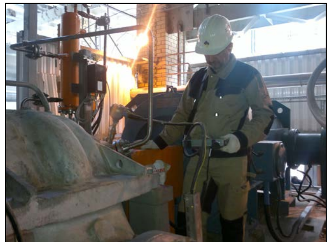
ITT Russia's diagnostics specialist takes vibration readings from the problem pump after its impeller trimming.
