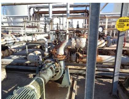
Original pump installation
