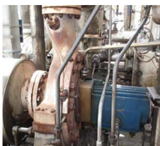
Original Non-Goulds Pumps equipment
