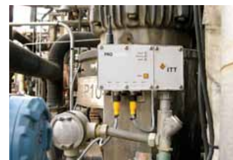
FIG 2. ITT installed its ProSmart system on the refinery's LVGO pump.
